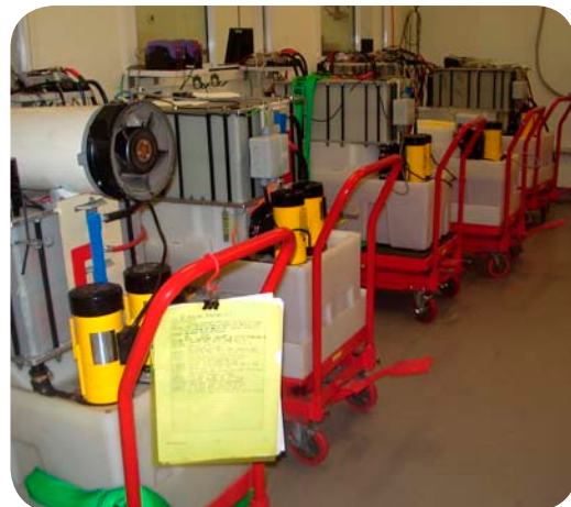
Photo 4. Units in test bay
