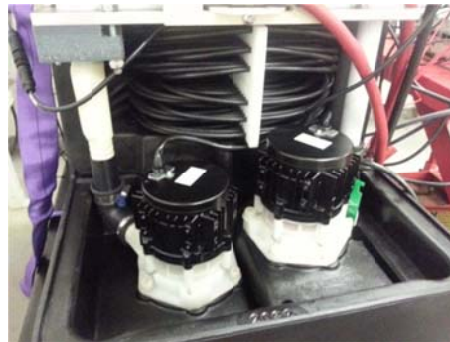
Variable speed DC pumps
