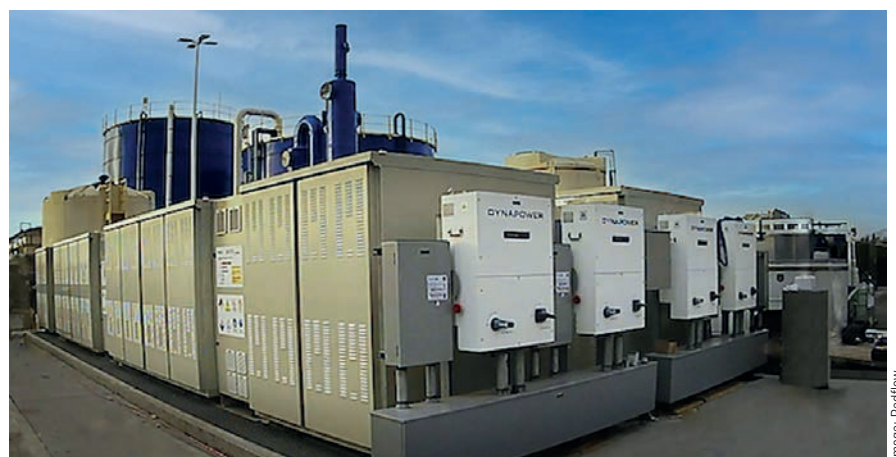
Fig. 3: 2 MWh of Redflow zinc-bromine flow battery energy storage and Dynapower inverters at the Anaerobic biogas facility, California.
